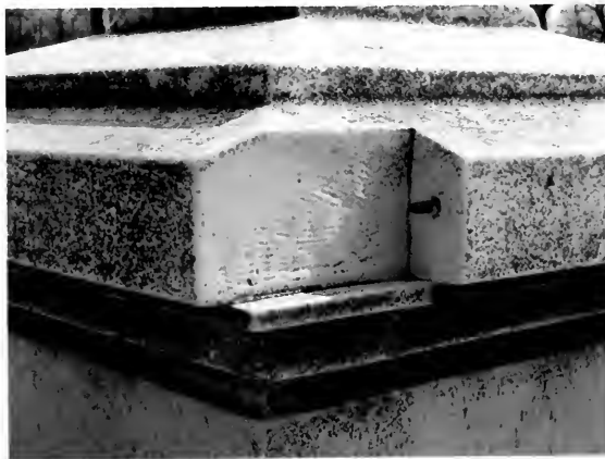
Figure 26: Missing dutchman repair and exposed metal pin
